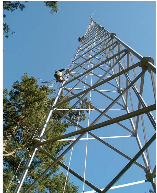
With the wind generator installation complete, it's time to begin installing the PVs.
